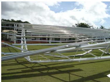
West Cairns Bowls Club roof collapse, legal reporting and expert witness
