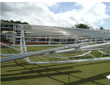
West Cairns Bowls Club roof collapse, legal reporting and expert witness
