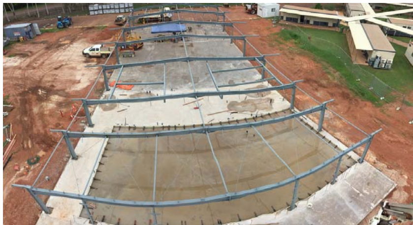
Design & Engineer of Rio Tinto sqm Mess Hall, Evans Landing near Weipa. Includes commercial kitchen, dining space & gym with 24/7 access. Under construction in 2017.
